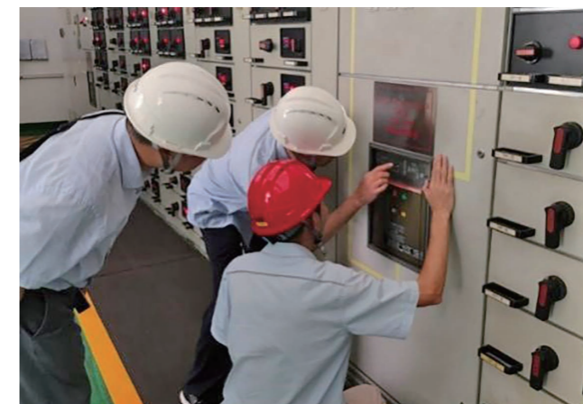
▲ 专家团队在南立 1-2 水电站做安全检查 The expert team is doing a safety inspection at Nam Lik 1-2 Hydropower Station
